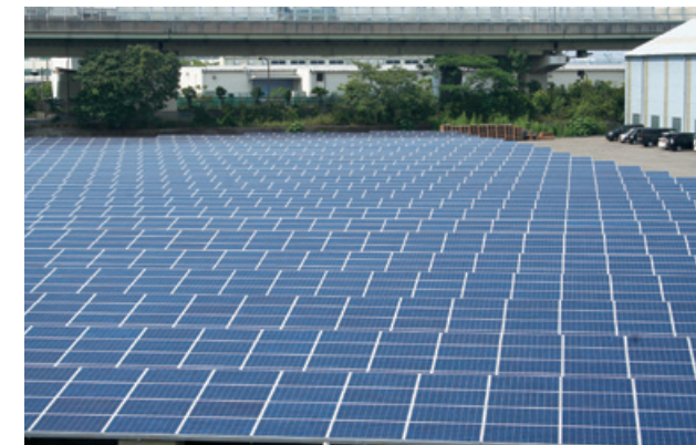
A solar energy system at the Izumiotsu Plant
