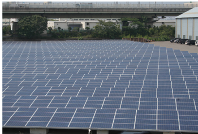
Solar panels at the Izumiotsu Plant
